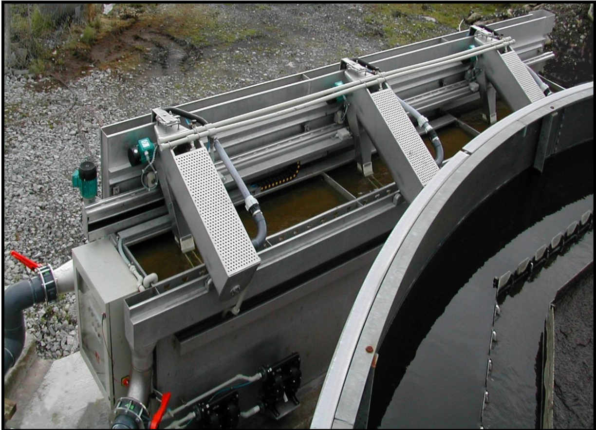
View from above showing the wash water pumps and secondary clarifier
