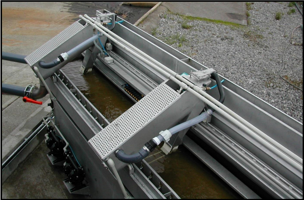
View down into the filter showing two of the sand washers
