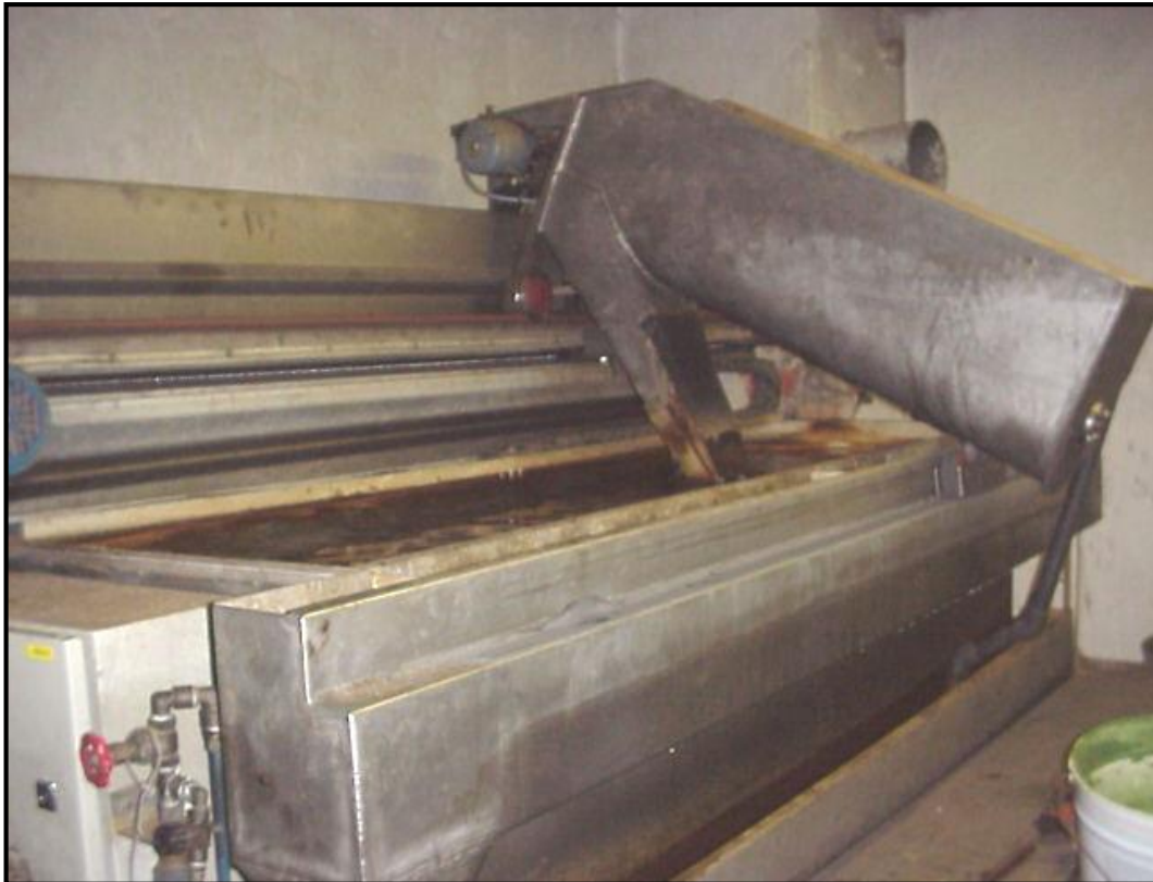
View of the TOVEKO filter
