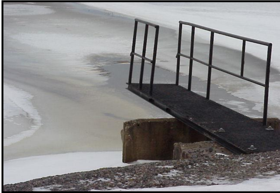
Influent pit to cleaning plant
