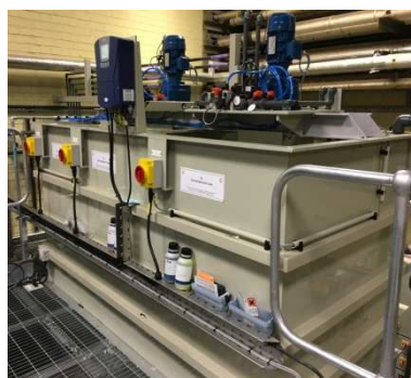
Chemical Treatment Stage
