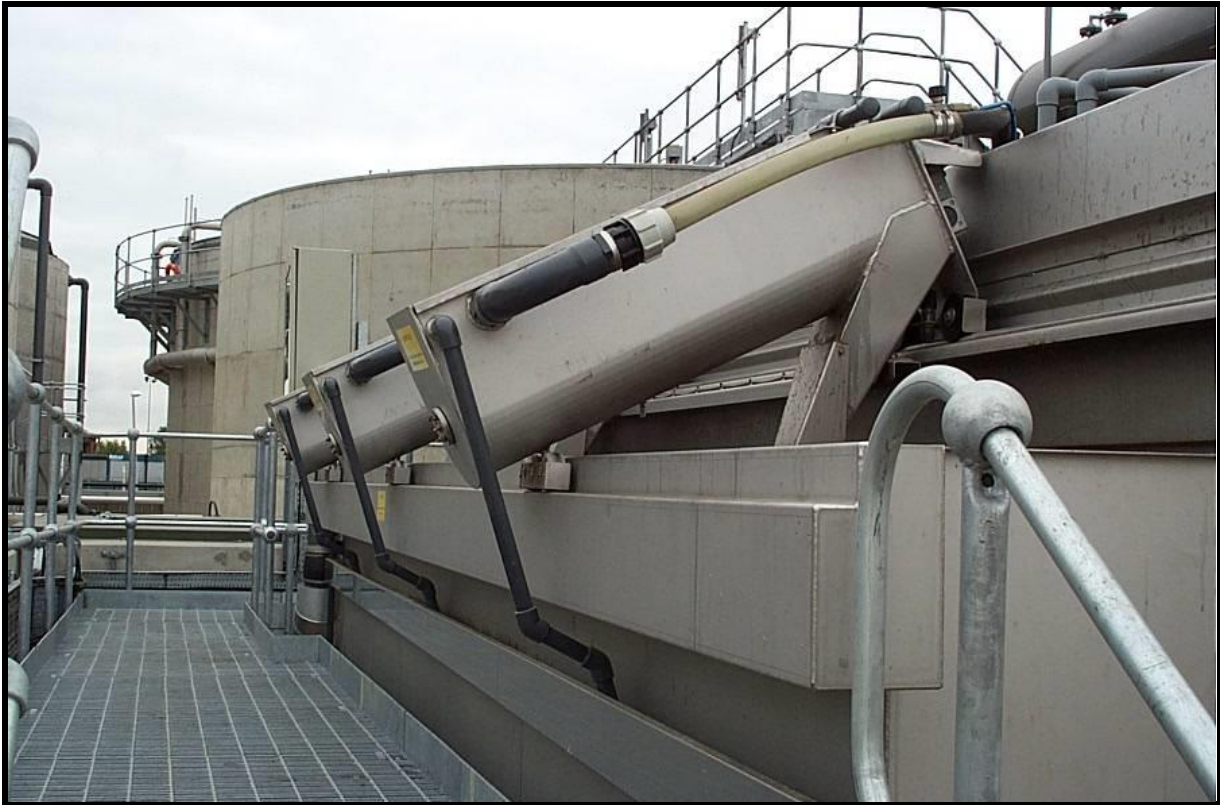
Filter view from ground level
