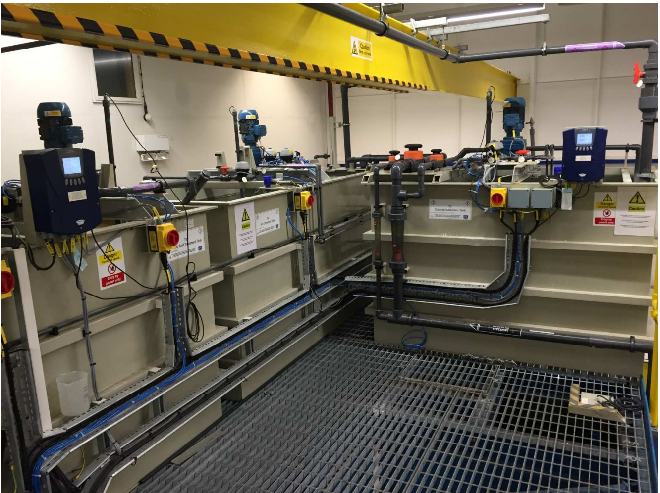
Chemical Treatment Tanks
