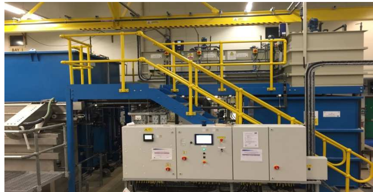
Plant general view showing control system
