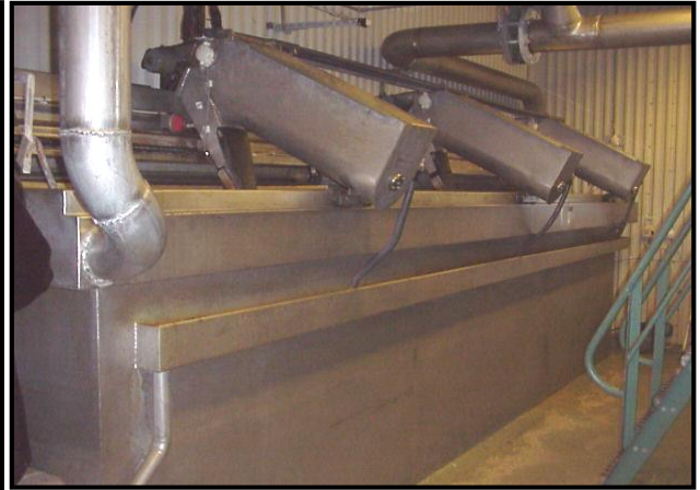
Toveko CX filter as final treatment stage
