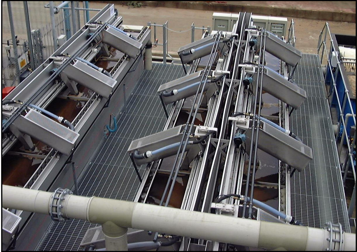
Top view of filters showing sand washers
