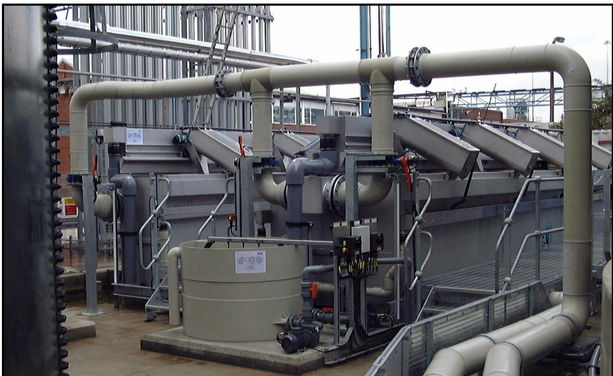
End view of the two filters showing the wash water supply system in the foreground
