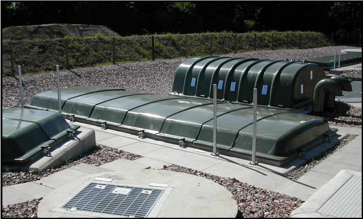
The sand filter is located below the long rectangular cover
