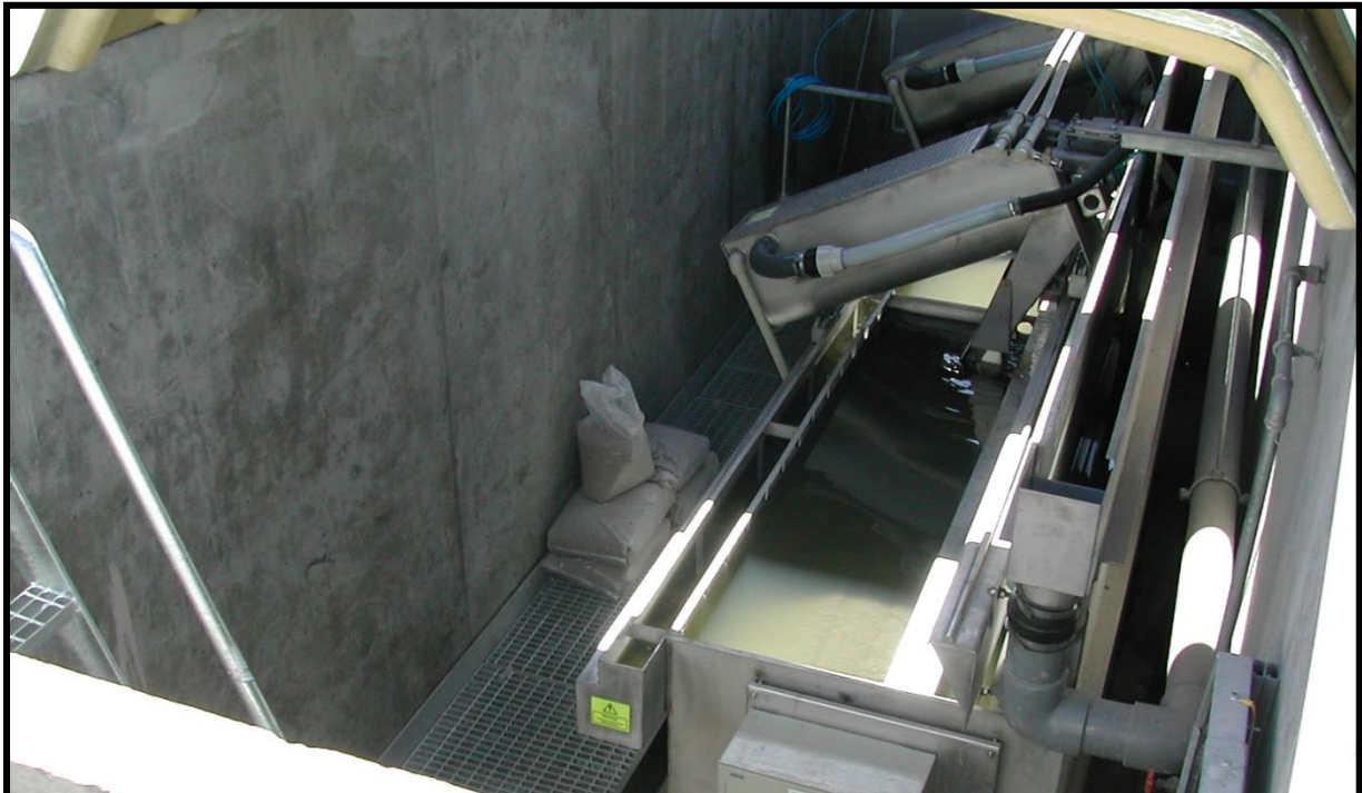
The model S-300 filter installed with the GRP covers removed
