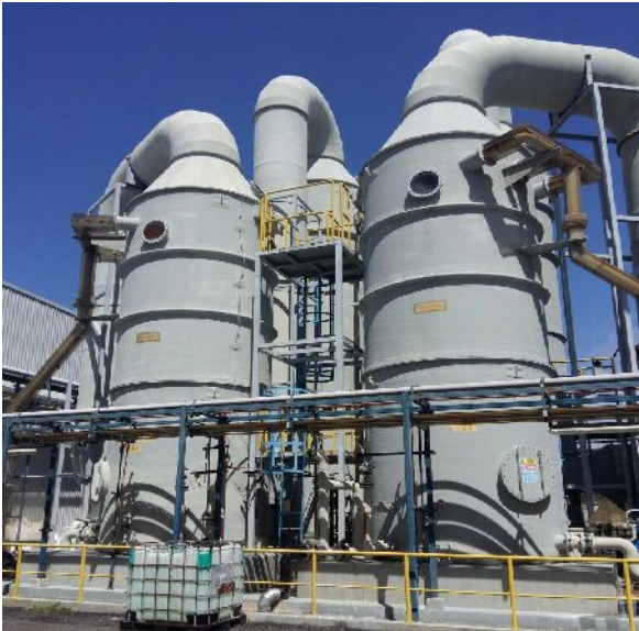
Ammonia Removal System
