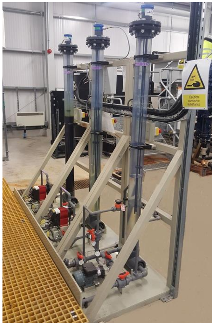
SecureChem™ IBC Automatic Level Control for three chemicals
