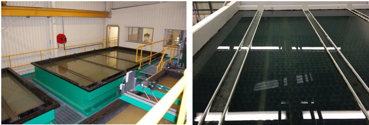
View down into H+E's highly-efficient Lamella Tube Settler tanks
