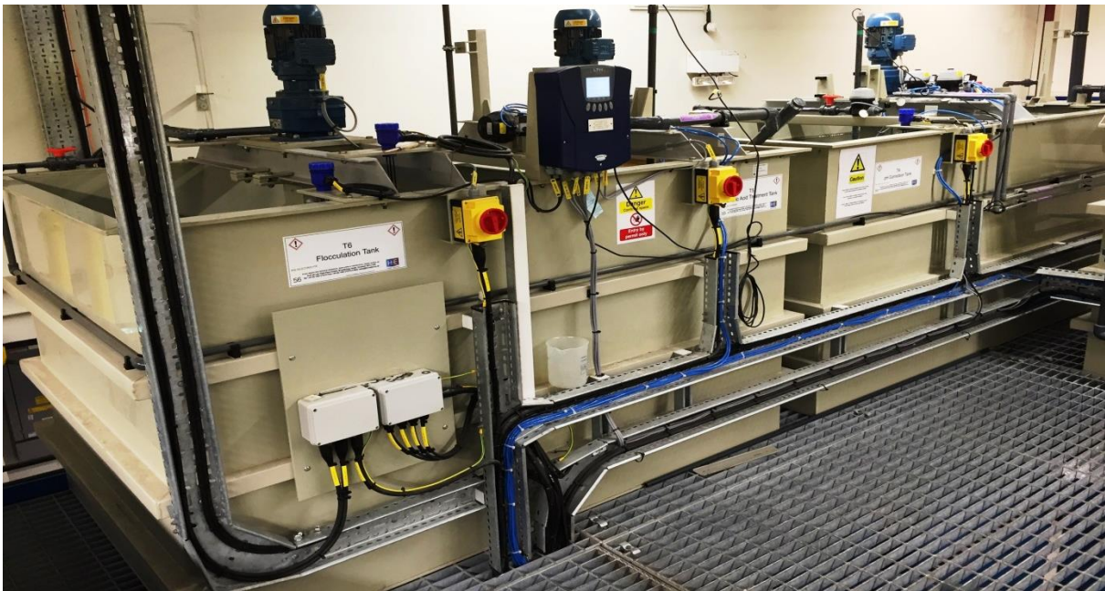
Chemical Treatment stages, all pre-assembled before delivery to site
