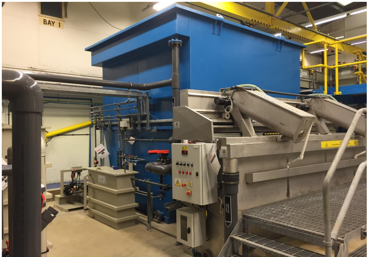
General view of a plant treating wastewater from metal finishing processes
